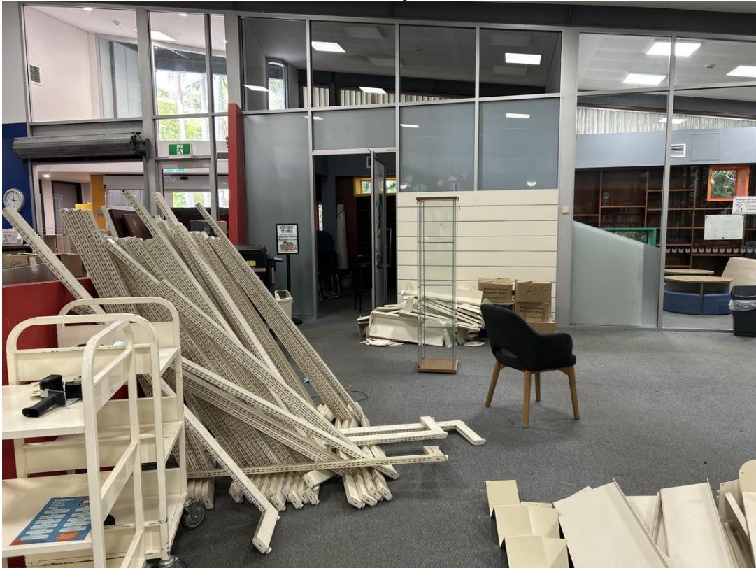
Image 3 Kingscliff Library during refurbishment: front public entranceway to the left under roller door, view of enclosed walls (where new children's area is now)
